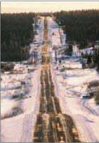
The Alaska Highway in winter is often covered in snow and affected by frost heave. Since it was opened to the public in 1949, teams of maintenance workers have ensured that the road is open year round.
